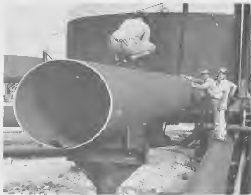
WORKERS ALONGSIDE and astride the 36-inch line indicate just how big the pipe is.
